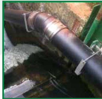
Pipe eel pass
